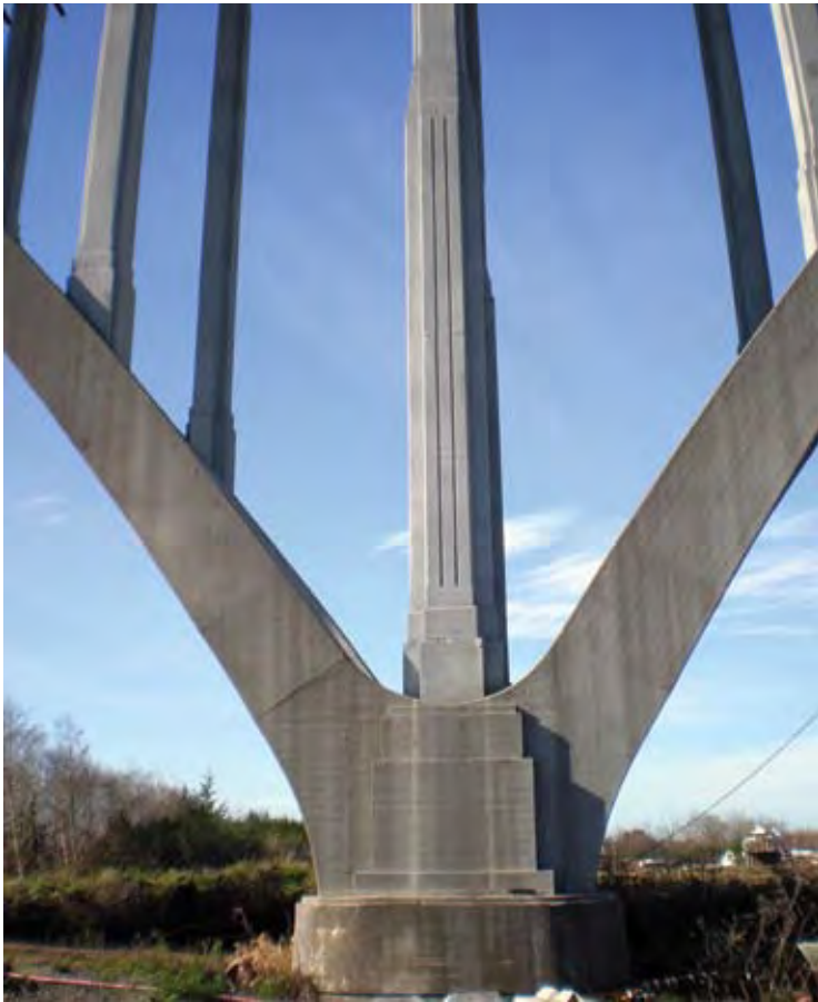
Inside the enclosure you could see the series of platforms that reached out to the center of the enclosure, which was currently erected around one of the main support columns. This photo shows the graceful sweeping nature of the design of this bridge. Note how the arches come together from either side to meet the column. The surface of the repairs has been sandblasted and coated with zinc as a part of the cathodic protection system
