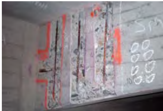
The repair has been prepared. Rather than cutting out reinforcing bar, the surrounding concrete is prepared and a box form will be built around it
