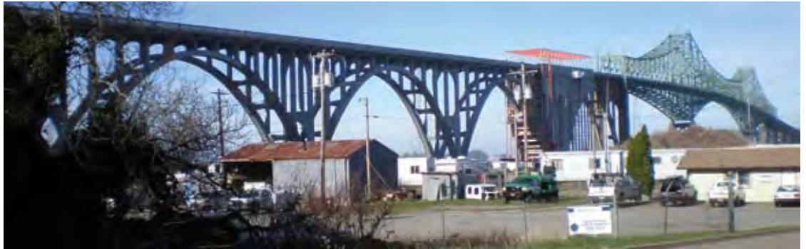
South end of the bridge. Enclosure is visible right before the steel midspan. Scope of work was to repair the South end, a 4-year project
