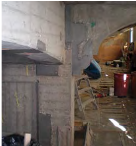
More complex, three-dimensional repairs can also be completed with the solution created by the team. Forming and pumping does not limit the repair to flat surfaces. Note the architectural corbel formed just right of center. Remnants of the white plastic tapit shells are still in the wall, used to hold the form in place
