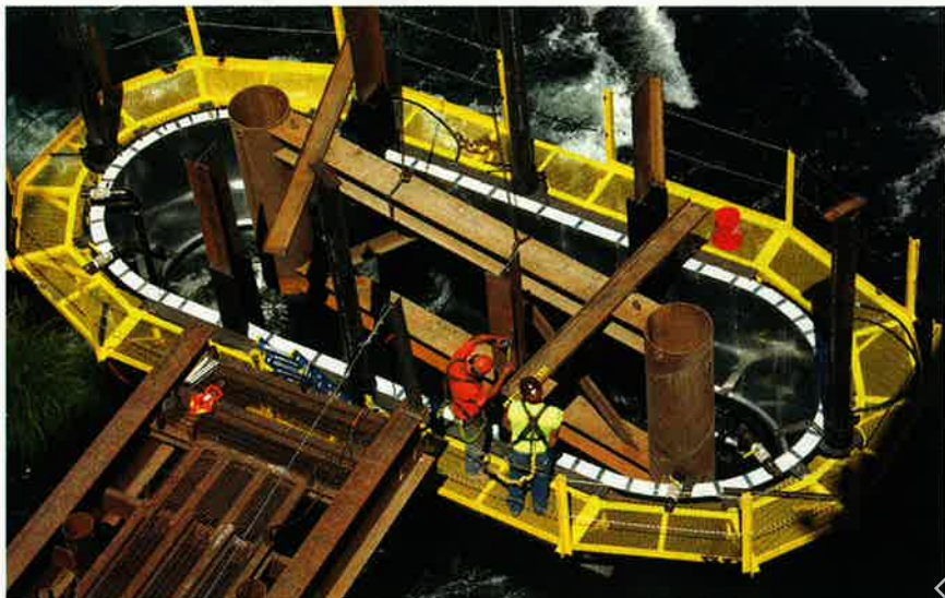
PEACEFUL PILE DRIVING Foam-lined platforms, a hydro-acoustic noise attenuator and compressors were used to minimize vibrations, create an air curtain and avoid disturbing fish in the Willamette River.
