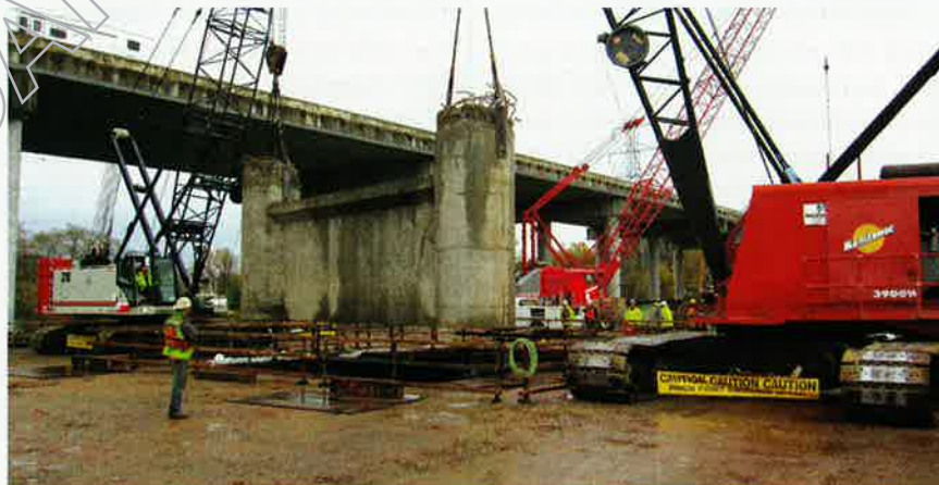
TEMPORARY BRIDGE AWAITS DEMOLITION Some slabs from the temporary bridge will be reused on the northern span of the permanent bridge as part of the project's environment-friendly nature.
